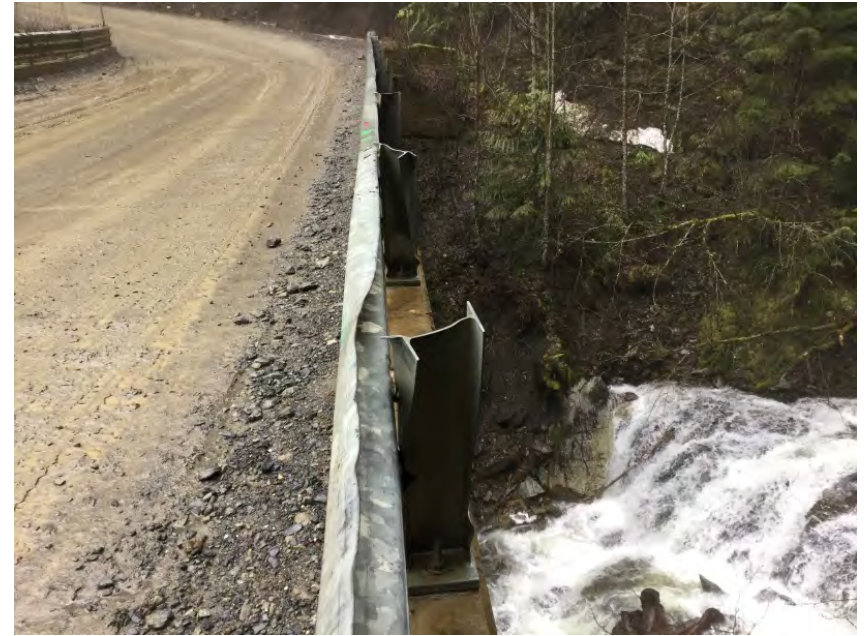
Damage to upstream risers - still functional
