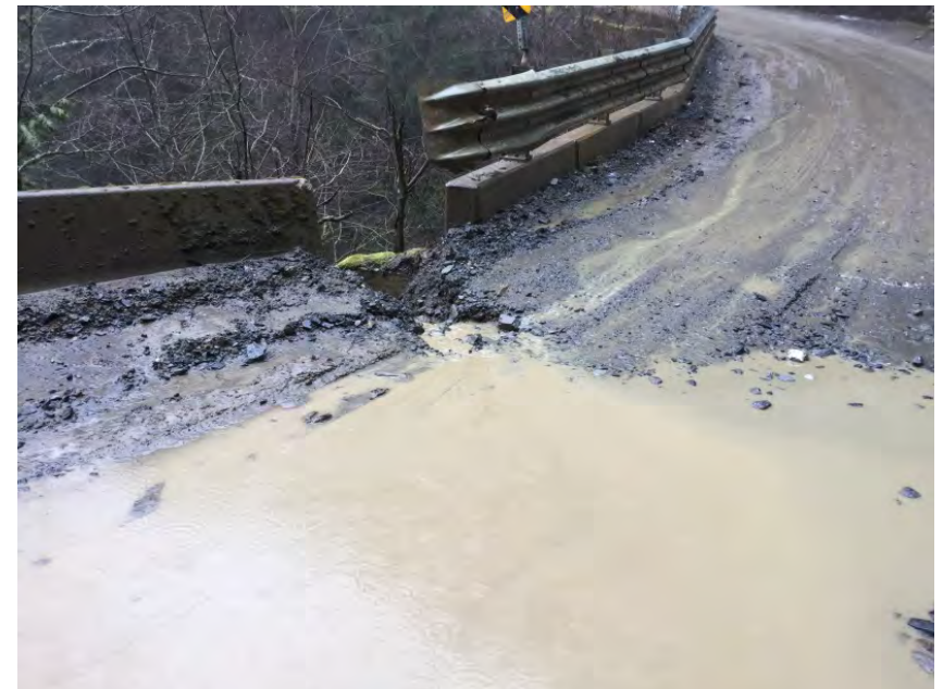
Eroding road surface at left downstream approach
