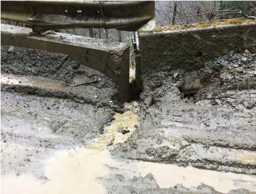
Eroding road surface and behind. ballast wall right downstream approach
