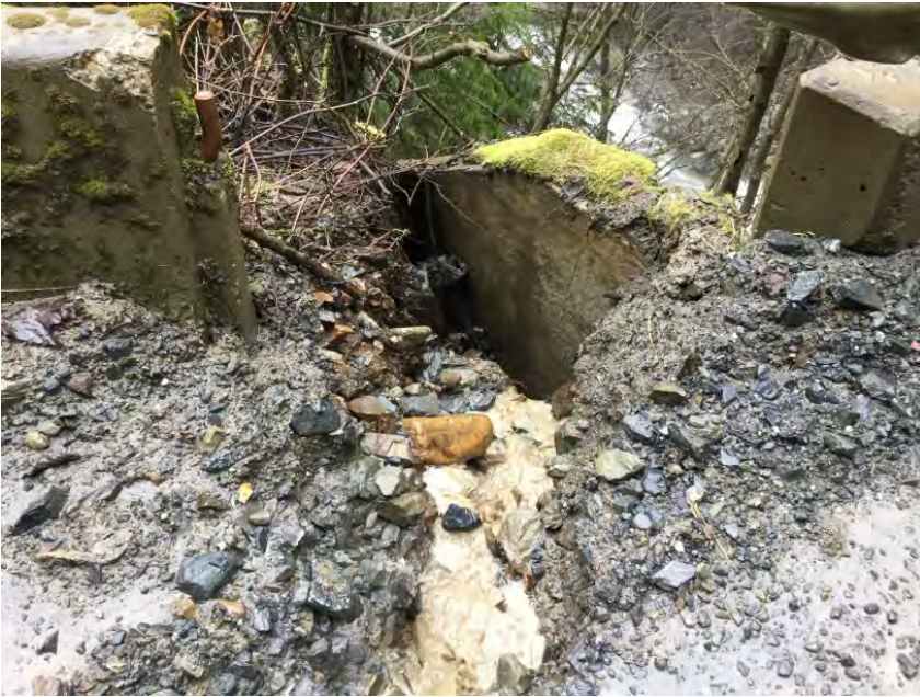
Eroding road surface and behind ballast wall on left downstream approach
