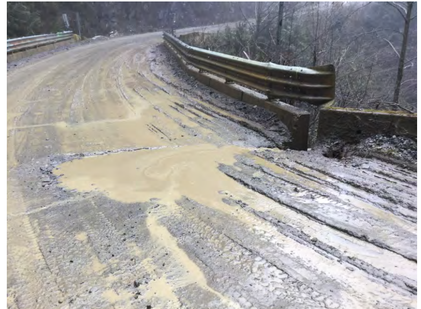
Eroding road surface right downstream approach
